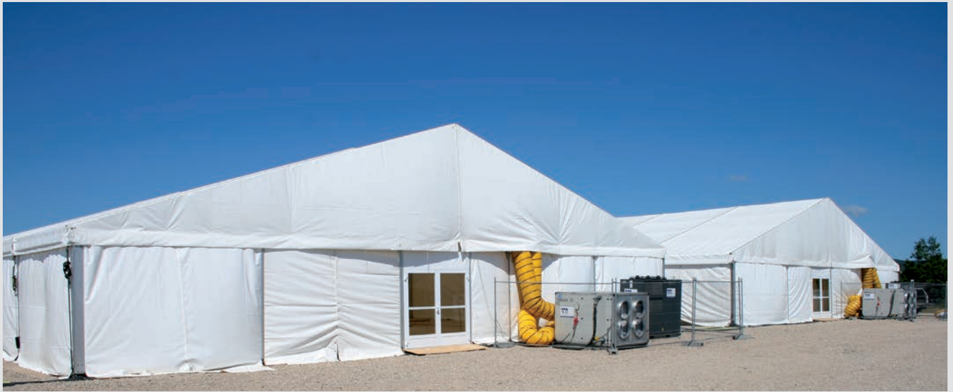
Large frame tents complete with lighting, electricity, air conditioning, and heating
